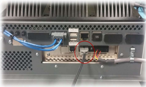
Figure 4 front panel fiber optic cable location
