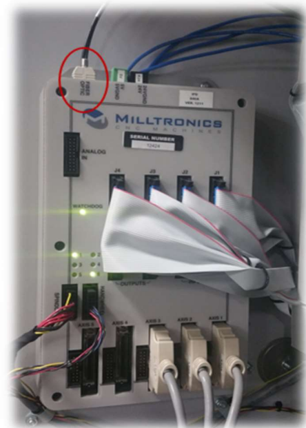
Figure 5 interface fiber optic cable location
