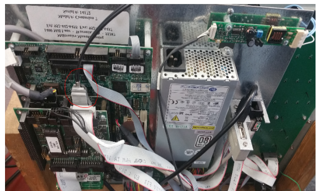
Figure 7 front panel fiber optic cable location
